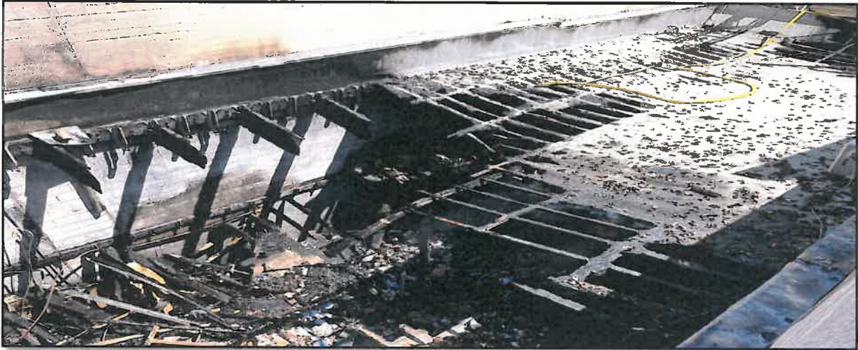
Perspective of roof from Bravo exposure looking back towards the Alpha side
