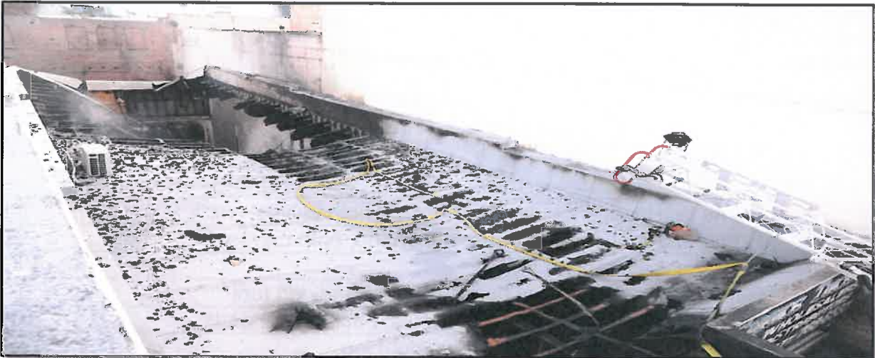
Perspective of roof from Bravo exposure looking back towards the Charlie side
