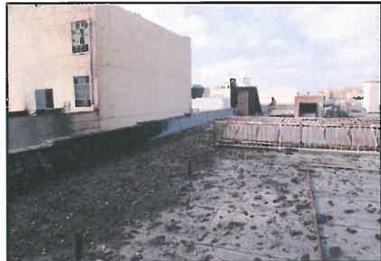
Nitrous Oxide Chargers on Bravo exposure roof
