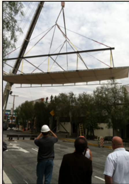
The mural protective shelter being lifted onto columns above the Italian Hall.
