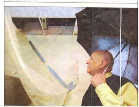
Zine shielding himself with an umbrella, checks the rain damage to the ceiling in his City Hall Office.
