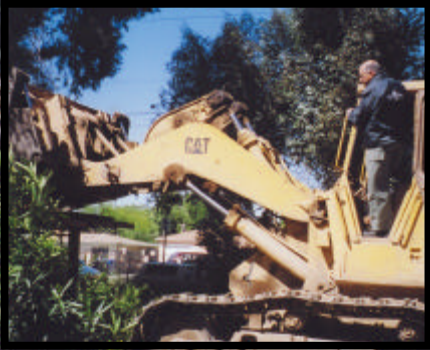
Councilman Dennis P. Zine on bulldozer demolishes a home used as a hangout for drug dealers and gangs.
