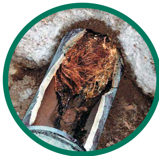
Photo shows tree roots that have grown into a sanitary sewer line and clogged and broke the pipe.
